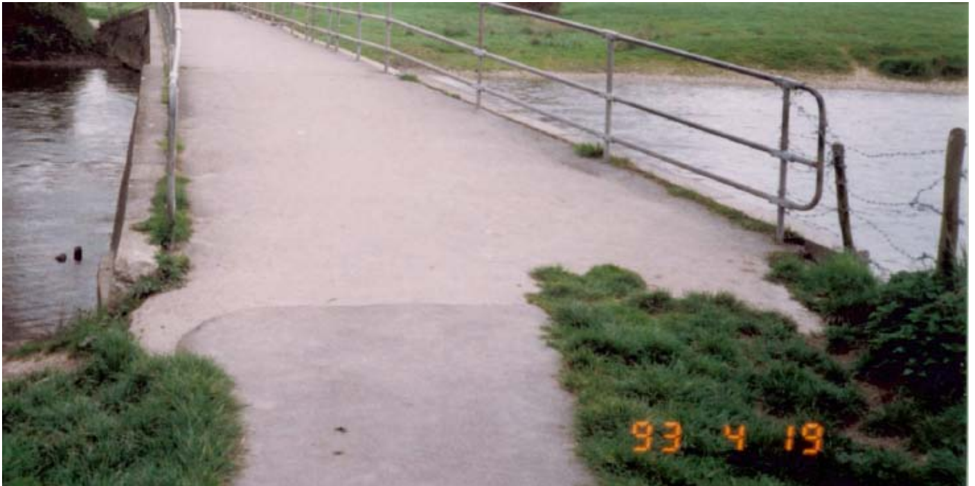
19 April 1993 The barbed wire field fence has been secured to the bridge rails at the claimed land side of the bridge.
